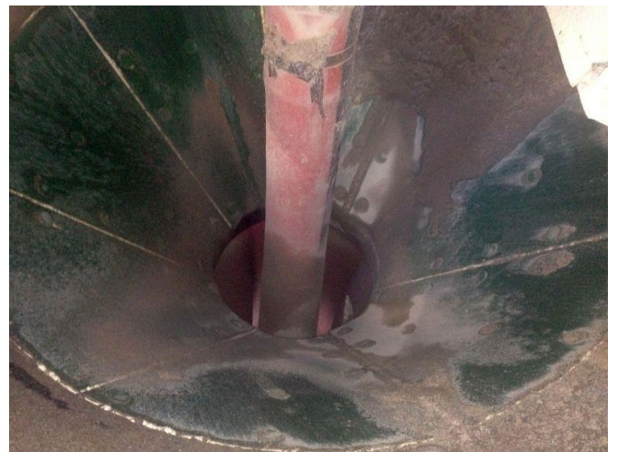
Same K-Superline® in Feb 2015, showing no signs of wear.
