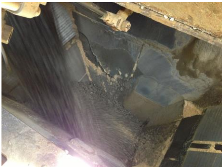
Photo of the internal sides of the hopper, showing the worn and uneven surface.
