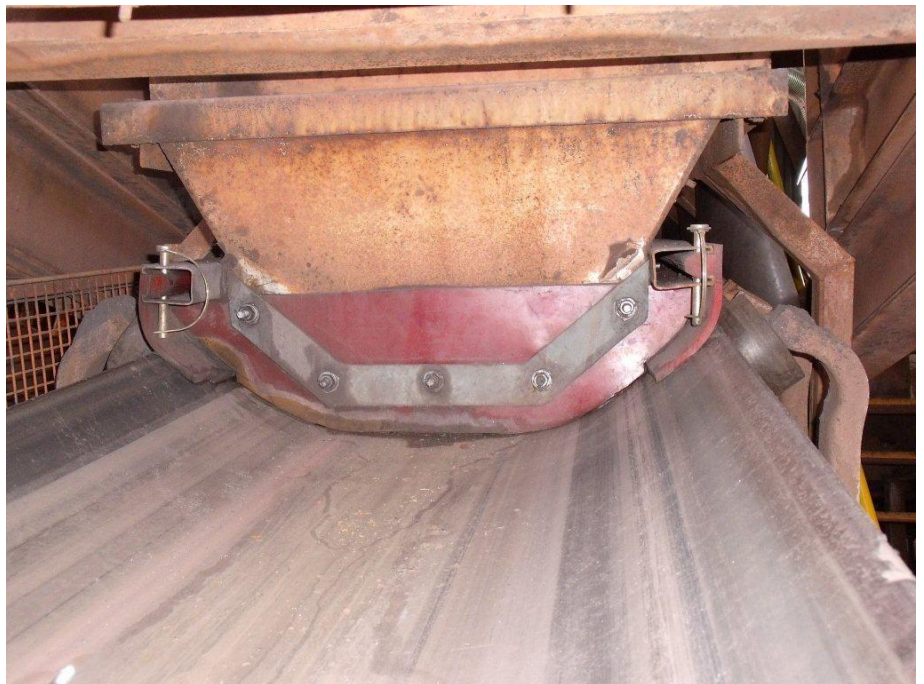
Full width photo of Port Pirie conveyor belt with polyurethane skirting K-Snap-Loc Dust Seal System.
