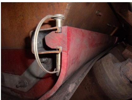
Detail photo of K-Snap-Loc Dust Seal System installed.
