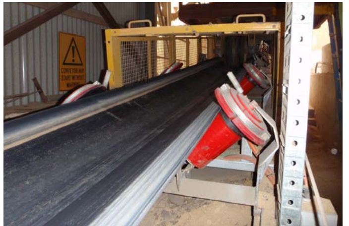
Images K-Sure® Belt Support and K-Superskirt® (top) and MTD Disc Tracker (bottom) in recent plant upgrades to conveyor equipment.
