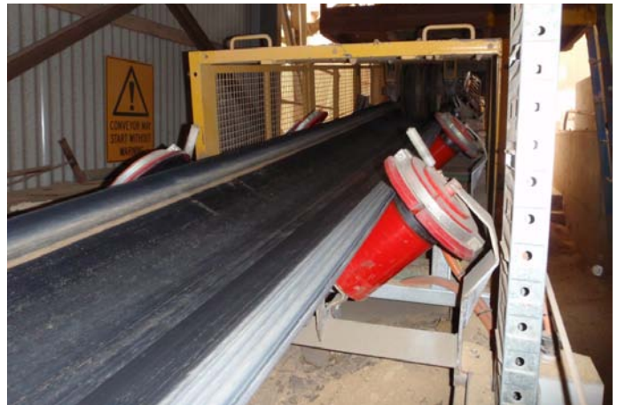
Images K-Sure® Belt Support and K-Superskirt® (top) and MTD Disc Tracker (bottom) in recent plant upgrades to conveyor equipment.
